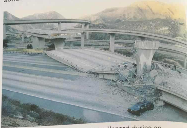
Figure 11.11 Part of this freeway collapsed during an earthquake near San Francisco. Part of it did not collapse because the concrete pillars had been reinforced to withstand an earthquake.
