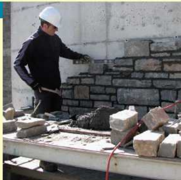
Jani Mroshaj uses a level to make sure the stone he just placed in this wall is straight.
